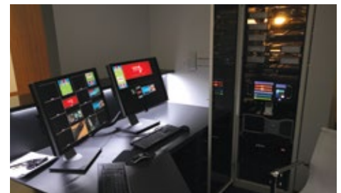
▲ Reduced rack space.
